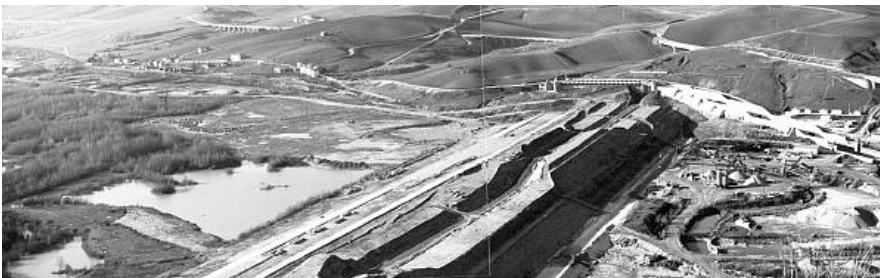
Figure 5.4 Conza della Campania dam during the construction of the embankment (www.prolococompsa.it and wikimapia.org). A lower height of the embankment is observed in the middle (section 4 of Figure 5.5).
