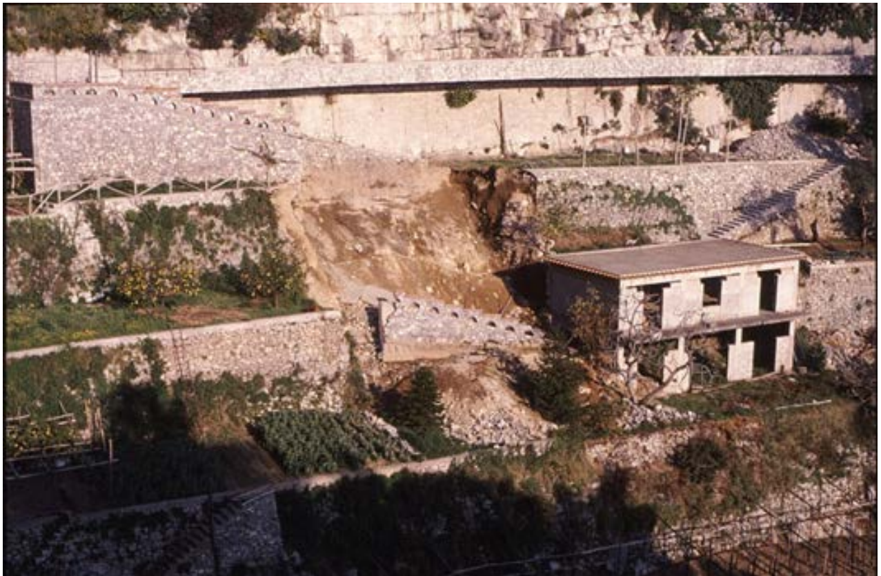
Figure n.158 - Typical landslide involving dry-stone walls on the Amalfi Coast
