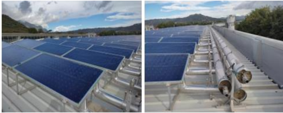
Figure 4.2 Solar Field test facility on the roof of TVP-Solar company
